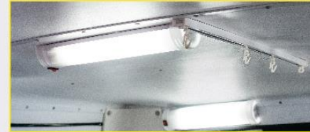
Roof lighting with transfusion bottle holders
