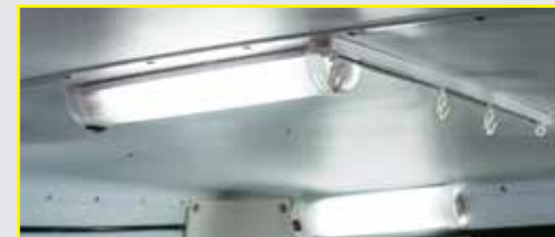
Roof lighting with transfusion bottle holders
